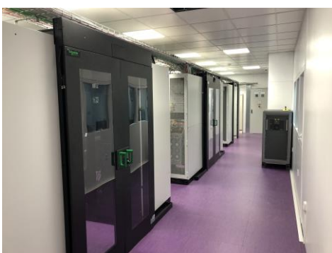
NetShelter Aisle Containment
