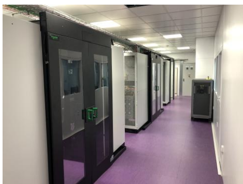
NetShelter Aisle Containment
