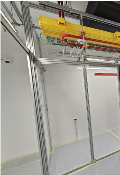
Hot aisle containment
