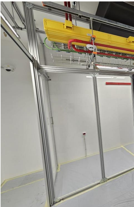
Hot Aisle containment
